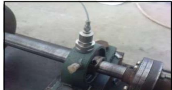
Figure 4: Transducer Installation Vibration Measurement Due to Imbalance
