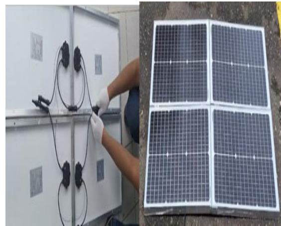
Gambar 12. Instalasi panel surya
